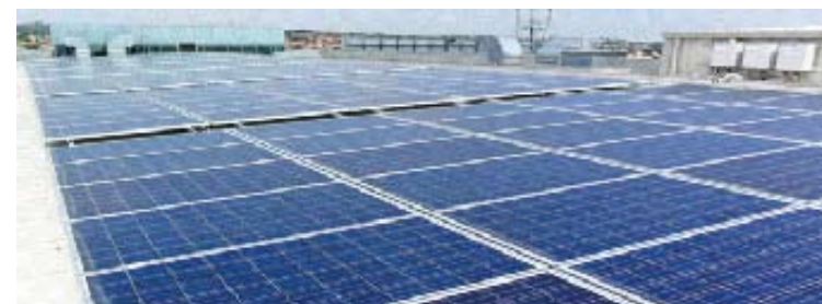
Photovoltaic System at the Data Processing Centre of Moncalieri
